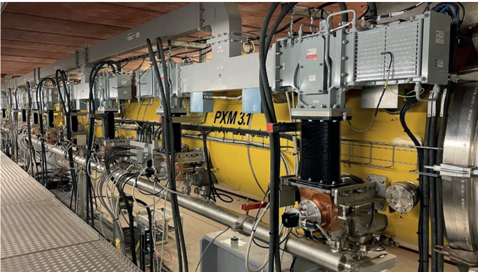
Figure 2 Module PXM3.1 (ACC3) installed in FLASH in 2022
