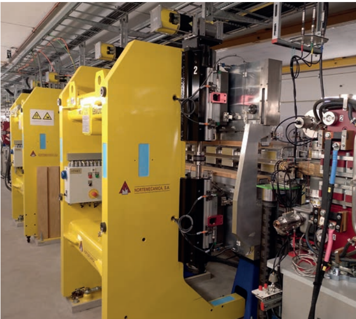
Figure 2 New undulator for the beamline P25 installed in the PETRA III tunnel
