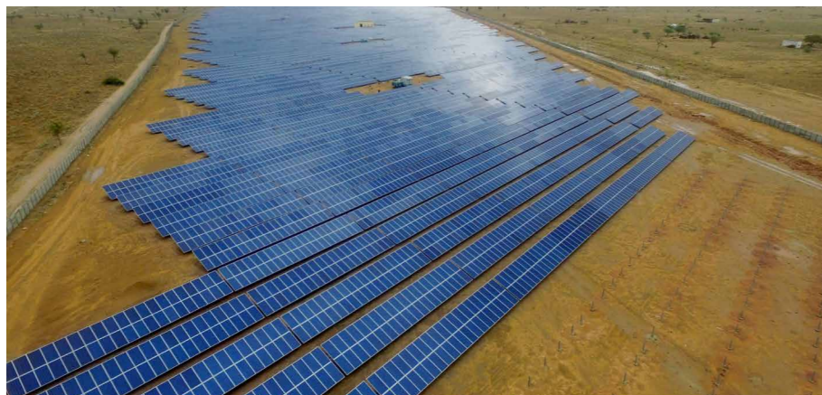
IBC SOLAR Projekt Phalodi in Rajasthan
