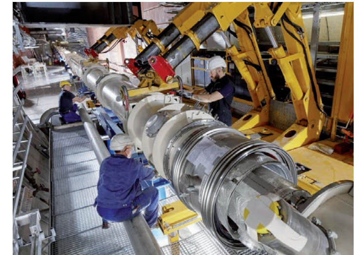
In late 2020, the last of the superconducting ALPS magnets were installed in the tunnel. Meanwhile, the entire chain has been cooled to -269^{\circ}\text{C} with liquid helium.
