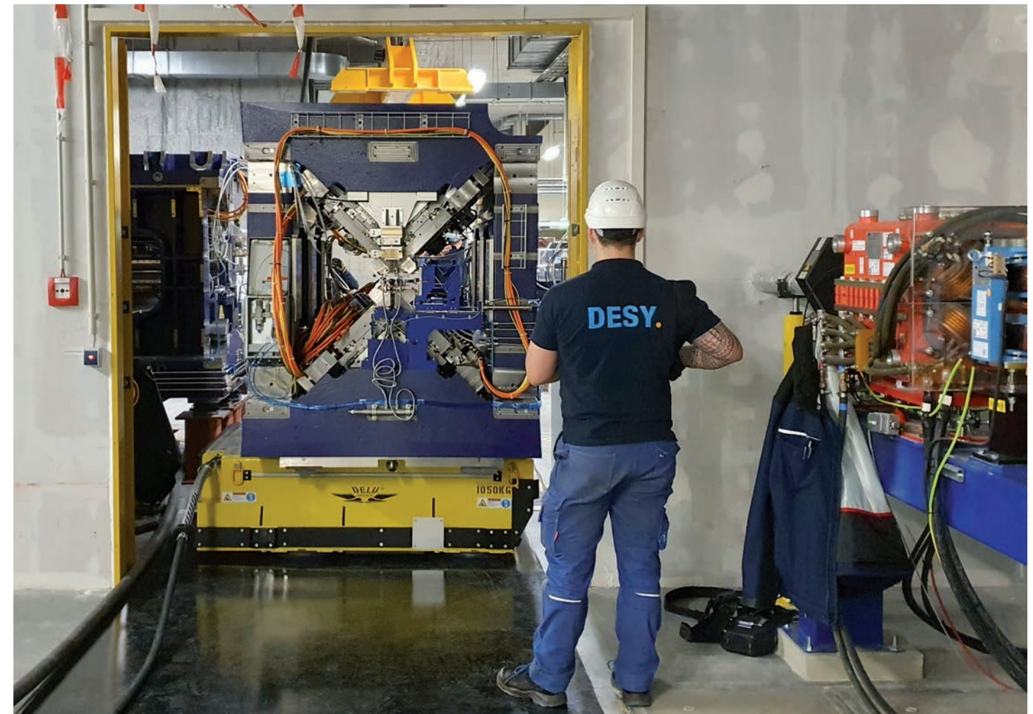
Figure 2 Transport of one of the APPLE-X undulators in the European XFEL undulator tunnel
