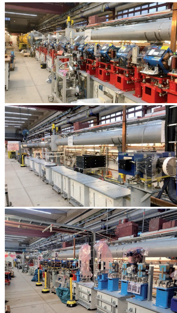
Figure 2 Ongoing refurbishment of the FLASH linear accelerator. The section downstream of the first bunch compressor and the ACC2 and ACC3 accelerator modules (top) were removed from the tunnel (middle) and are being replaced by a new first bunch compressor with laser heater and by European-XFEL-type accelerating modules (bottom), allowing for a higher accelerating gradient and thus shorter photon wavelengths.
