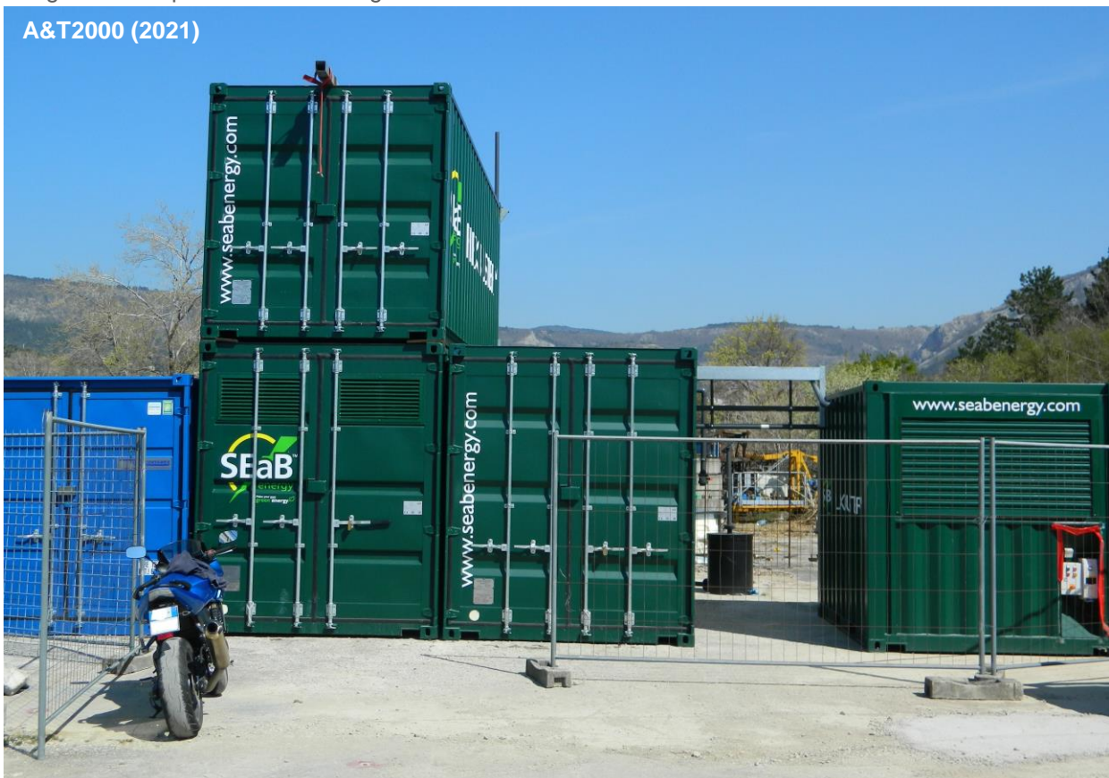
Figure 13: Micro-anaerobic digestion plant in Dolina. In process order from right to left: Biowaste reception unit, control unit, digester unit with gas storage unit on top, CHP unit (blue, Stirling engine) for energy generation
