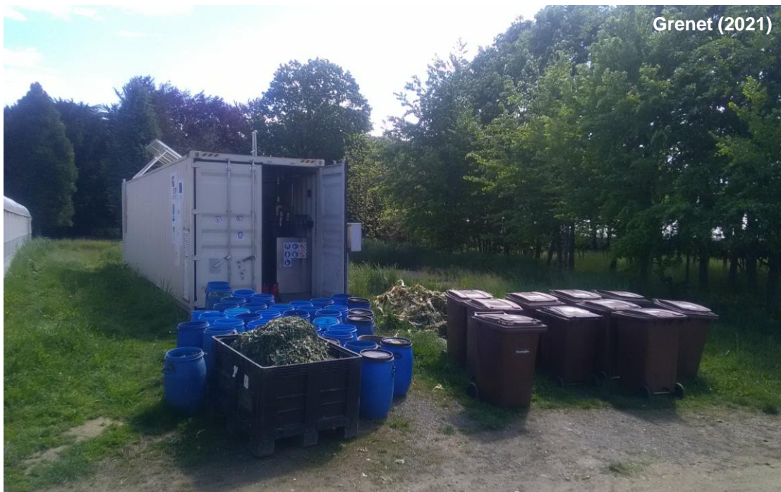
Figure 7: mAD unit of the Lyon demonstration site including FW storage devices
