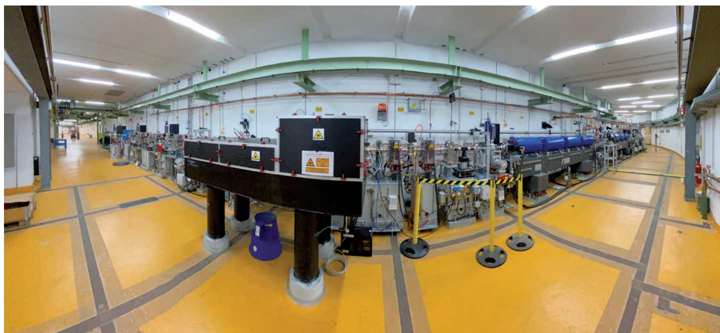
Figure 1 Panoramic view (“fisheye” representation) of the ARES linear accelerator installed in the former DORIS tunnel (installation status at the end of 2020). The gun area is to the right, the experimental area in the middle, and the beam dump to the left.
