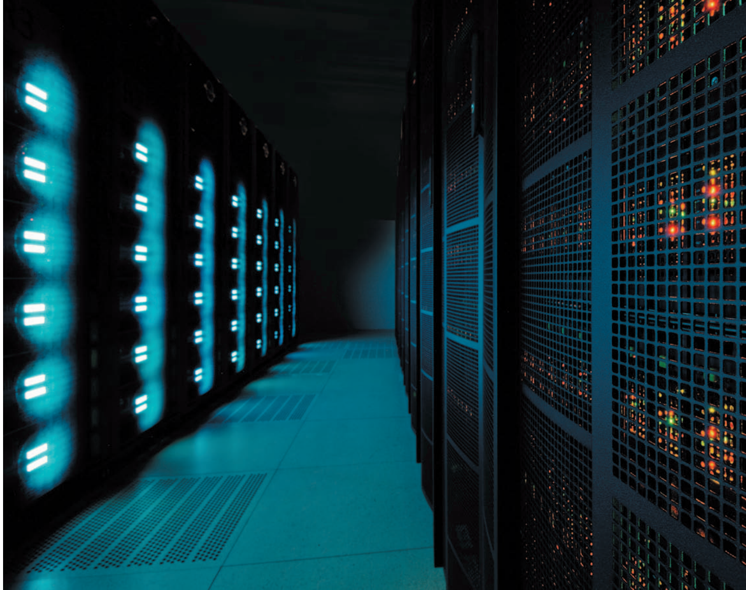
With the second stage of expansion in 2016, Mistral consists of ten such rows of computer racks – part of the hard-drive system (left) and the computational nodes (right) can be seen in the image above.
