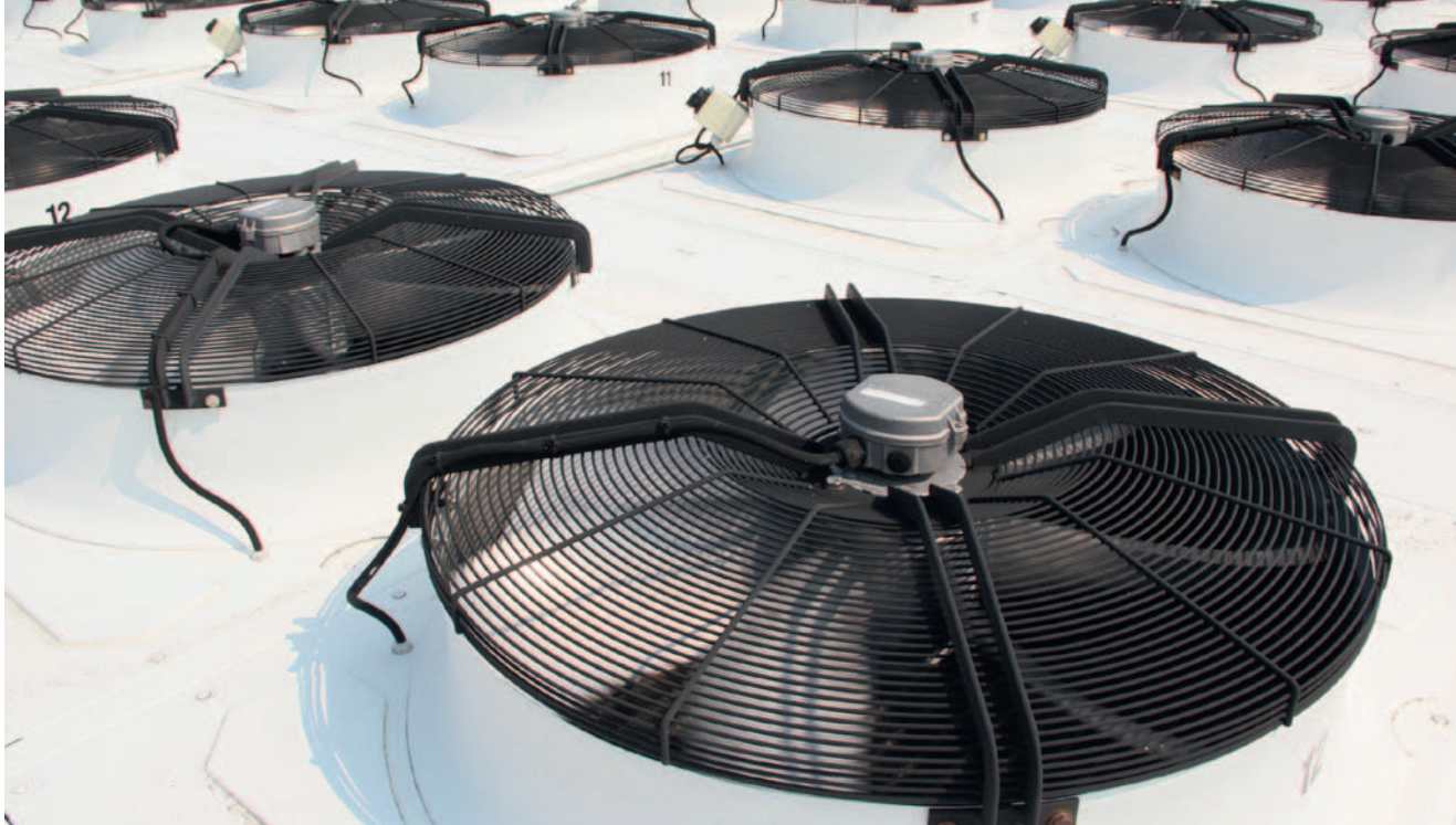
Fans are installed on the roof of DKRZ. They expel the heat produced by the computer to the outside.
