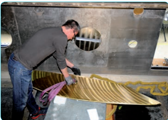
Fig. 1: Installation of the 1.8 m long full scale propeller tip at the side wall of HYKAT
