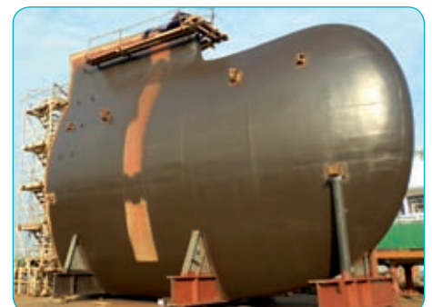
Photo 5: ES-Bow building block on the shipyard ready for first vessel to dock
