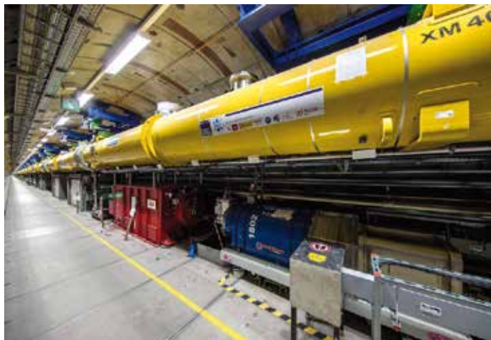
View into the 2.1 km long accelerator tunnel of the European XFEL with the yellow superconducting accelerator modules hanging from the ceiling
