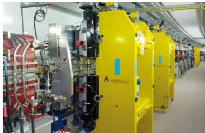
Figure 1 Three new undulators for beamlines P22, P23 and P24 were installed in 2017 in the Ada Yonath experimental hall.
