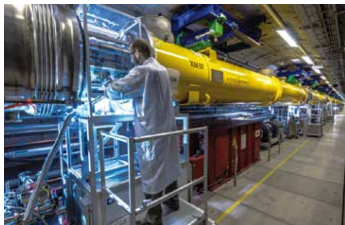
Figure 1 Connecting the beam vacuum systems of two superconducting modules of the European XFEL linear accelerator, using a small, localised cleanroom
