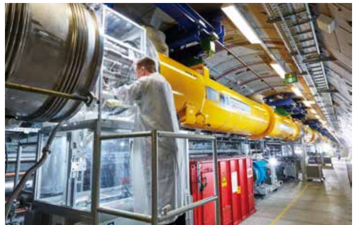
Connecting two accelerator modules in the European XFEL tunnel
