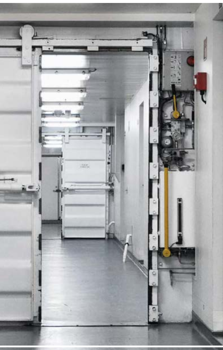
In an emergency, the proper use of power-operated watertight doors may save lives and assets.
