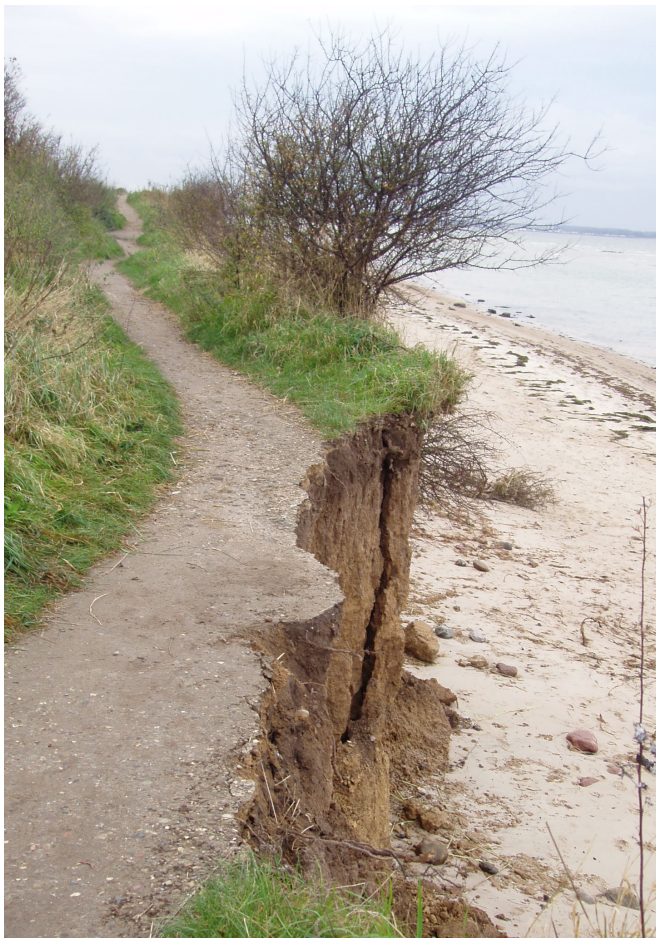
Accelerated erosion near Baltic coastline results in damage to infrastructure. Credit: Horst Sterr
