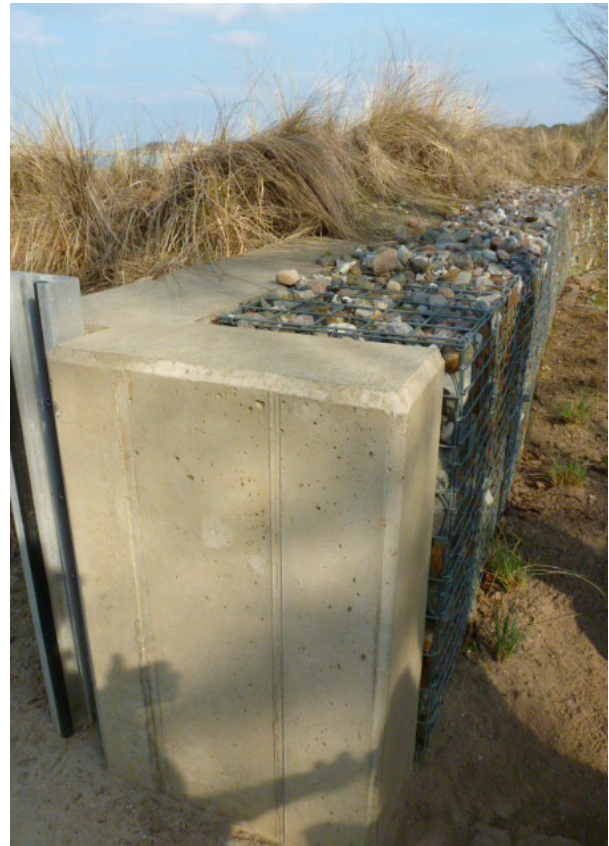
After nearly a decade of planning and discussion between community members, scientists, and regional officials, the coastal resort community of Timmendorfer Strand completed a sea wall. In many places the structure blends into the natural landscape, thereby minimizing aesthetic impairment while protecting the community from the impacts of storm surges. Credit: Susanne Moser.
