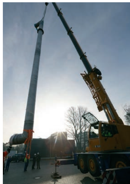
Figure 5 Another vertical cryogenic transfer line (February 2014)
