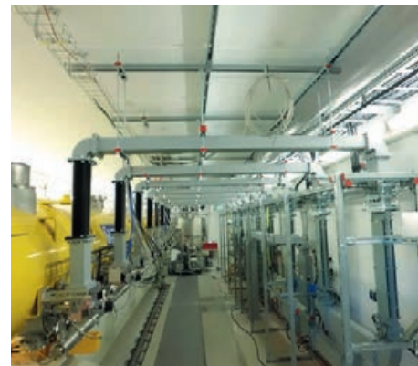
Figure 5 Installation of the RF waveguide distribution at the AMTF
