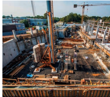
Construction site of one of the new experimental halls for the PETRA III extension, Hall North
