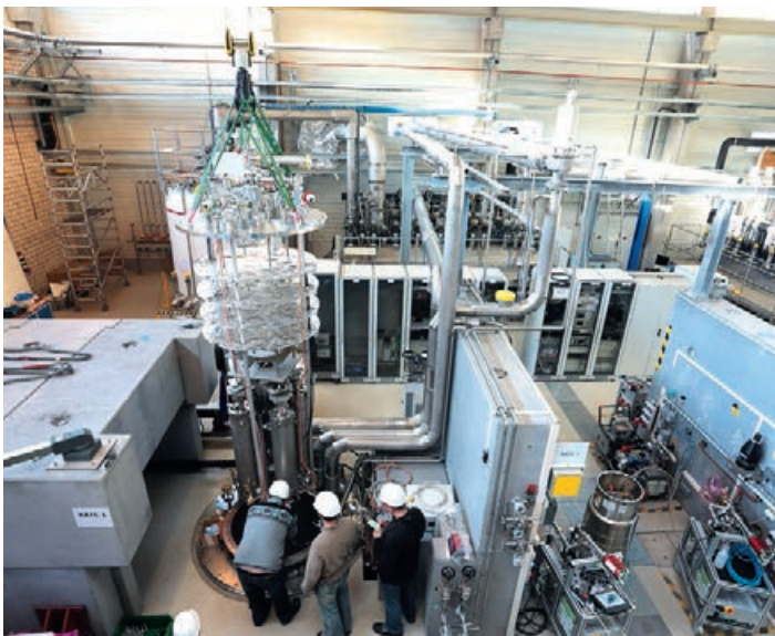
Figure 1 Vertical test stand with bath cryostat, concrete shielding and cryogenic installation at the AMTF. A cryogenic insert with four superconducting accelerating cavities is under installation.
