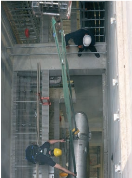
Figure 4 Inserting a vertical cryogenic transfer line into the media shaft in the European XFEL entrance shaft (May 2014)
