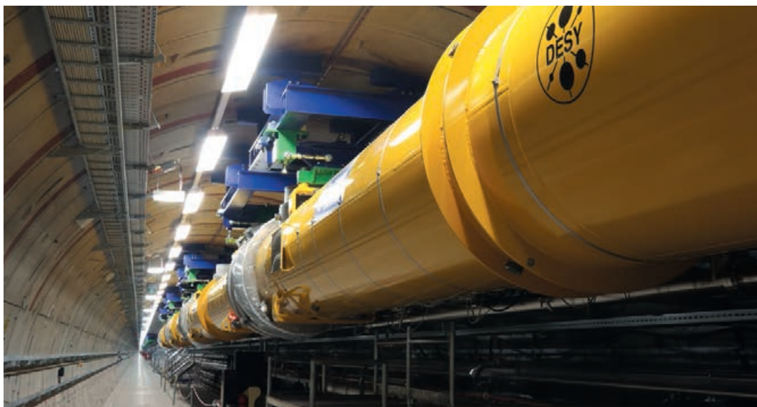
View into the main tunnel of the European XFEL X-ray laser with first accelerator modules
