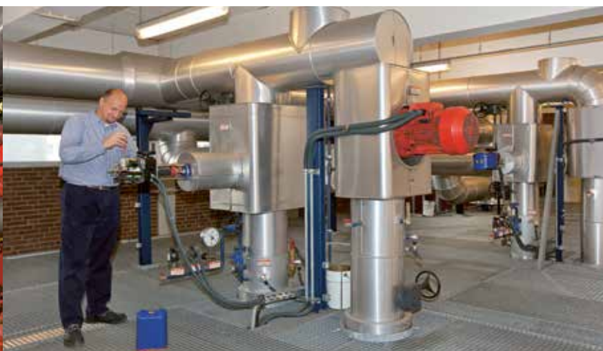
The central heating plant supplies heat to the southern area of the airport
