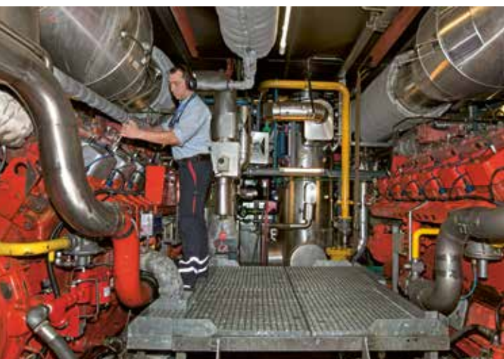
The power-heat coupling of the block-type thermal power station (BHKW) gives it a high level of efficiency
