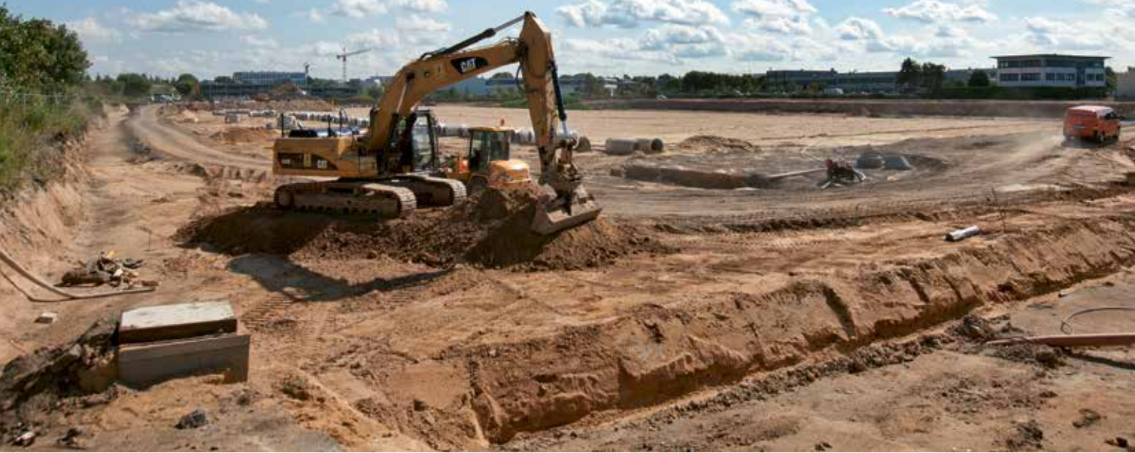
The new cargo terminal is taking shape on the site of the former remote P8 car park
