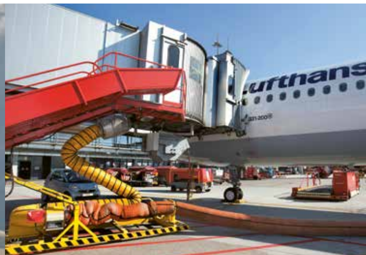
At Pier parking positions, the aircraft are supplied with electricity and air conditioning from the block-type thermal power plant and the APU remains switched off
