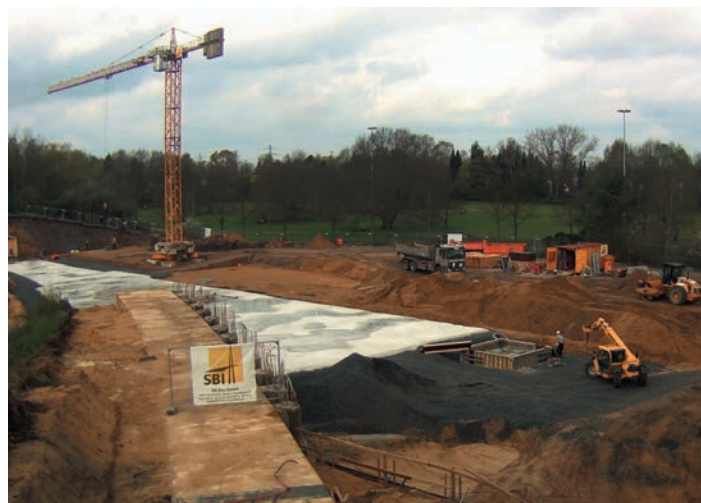
The civil construction work for the PETRA III extension hall North started with removing the soil that covers the storage ring tunnel in that area.
