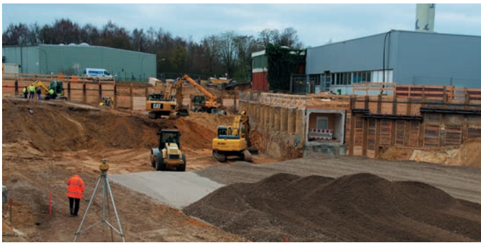
Figure 6 Digging at the site of hall east. The remaining tunnel is seen on the right (March 2014).
