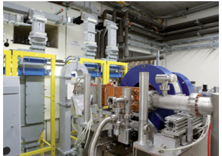
Figure 4 Four isolators with RF power waveguide combination (rear) and RF gun (front)
