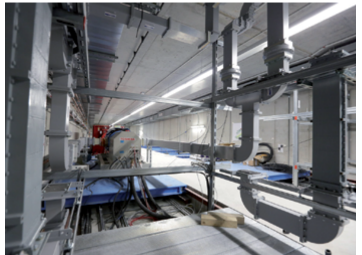
Figure 2 Toshiba E3736H multibeam klystron and connected waveguides
