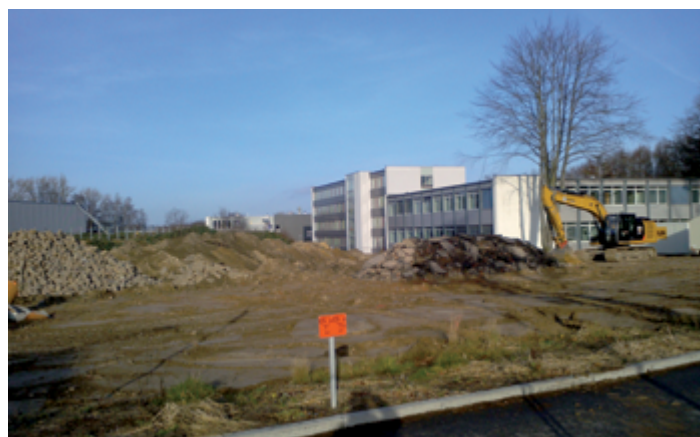
Figure 5 View of the construction site for the PETRA III extension hall East
