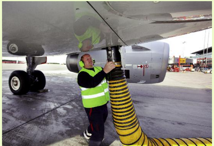
At Pier parking positions, the aircraft are supplied with electricity and air conditioning from the block-type thermal power plant.
