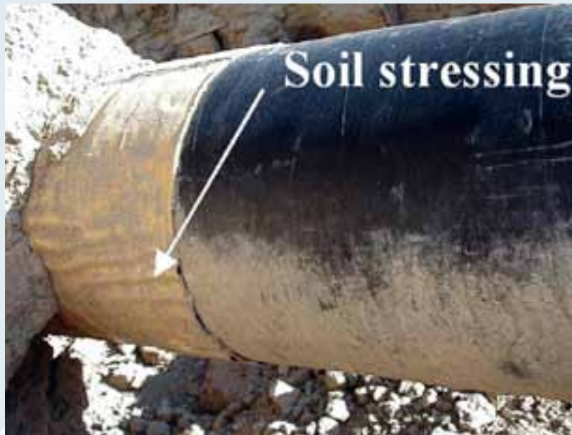
FIGURE 7. Soil stressing of an HSS at elevated temperature service.
