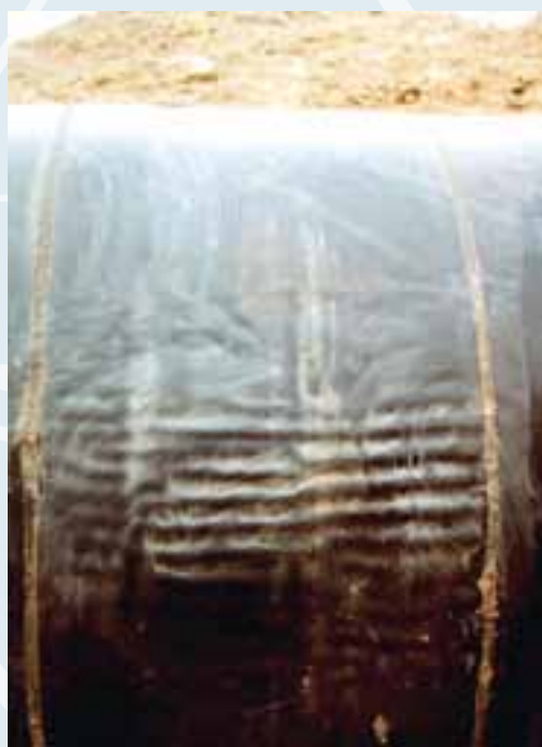
FIGURE 6. Wrinkling of HSS under the influence of soil loading and stressing.
