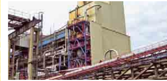
PLANT. The BGL gasification technology is one of the most efficient coal gasification processes available.
