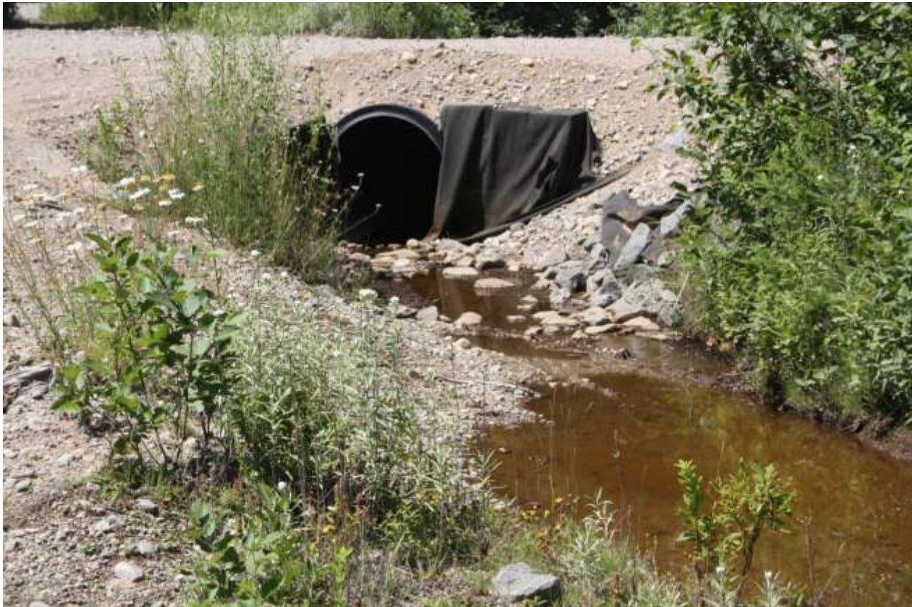
Figure 11: Creek Crossing in Tioweró:ton Showing Erosion Problems
