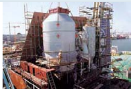
EXHAUST. Wet scrubber systems reduce SO x emissions.
