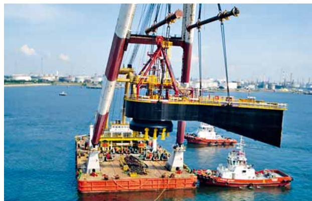
HEAVY LIFTING. FPSO vessels must be anchored reliably. The technology preferred today is a single-point mooring (SPM) system.
