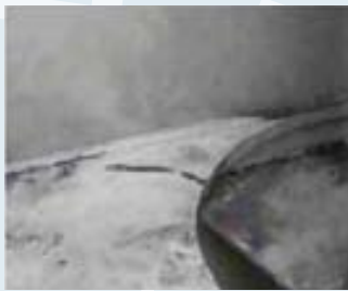
FIGURE 7. Typical hatch-corner crack damage.
