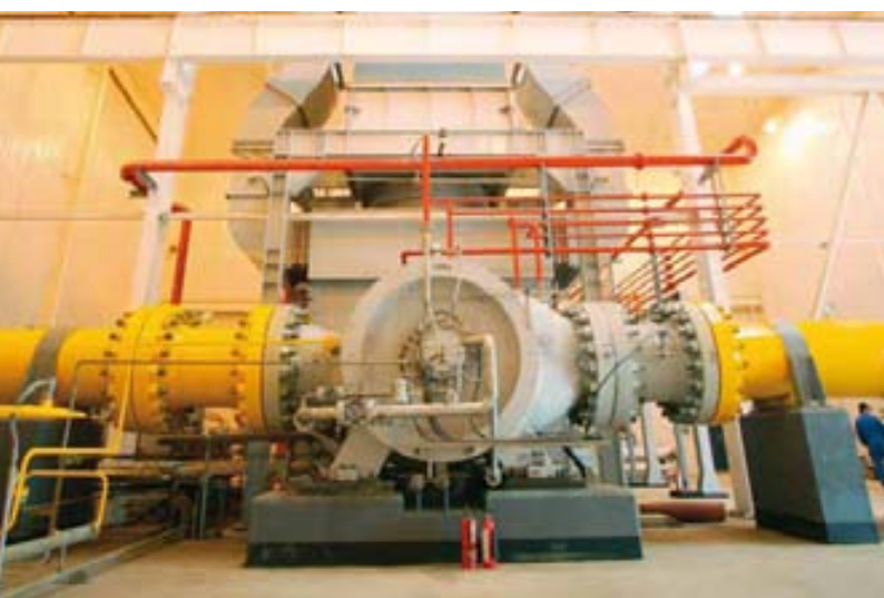
COMPRESSOR STATIONS. Optimization reduces energy consumption.
