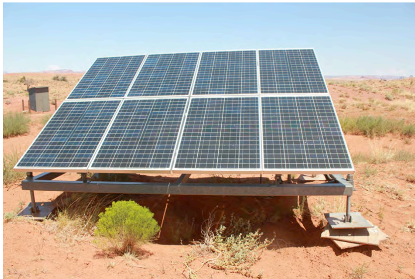
Figure 10. The high winds during an extended drought period have eroded the land surrounding the foundation of a PV system. Photo taken by Dr. Stanley Atcitty.
