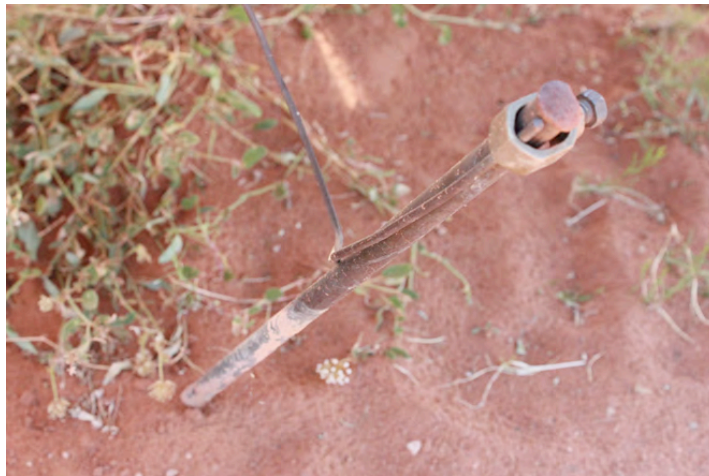
Figure 13. Grounding rod that has been exposed more than two feet above ground due to the extended drought in Arizona causing increased dust storms and erosion. Photo taken by Dr. Stanley Atcitty.
