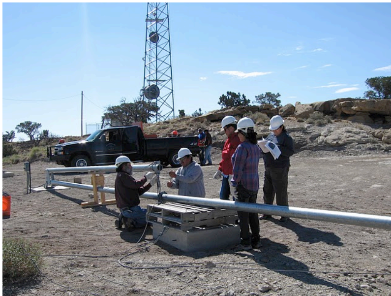
Small wind turbine workshop hosted by Navajo Technical College Photo credit: Sandra Begay-Campbell
