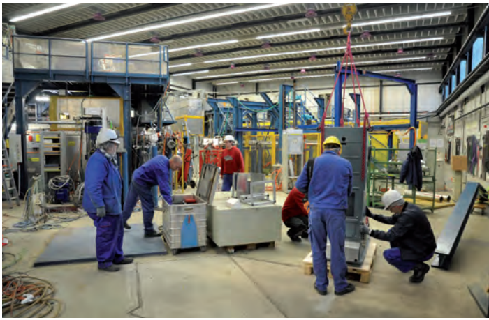
Figure 3 Right after the shutdown, beamlines and instrumentation at DORIS are being dismantled and removed.
