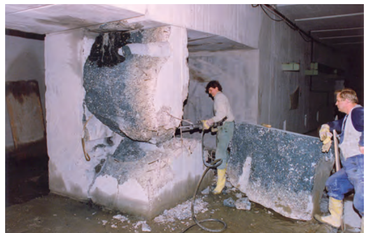
Figure 5 “Paving the way” in the DORIS II ring tunnel to accommodate the “bypass” (Fall 1990).
