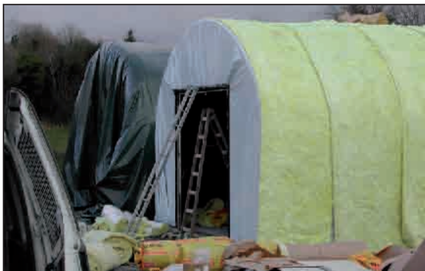
Plate 8.2: The construction of a new Perch broodstock facility at PDS, Ireland. Three layers of insulation provides very efficient heat retention, thereby reducing energy costs.
