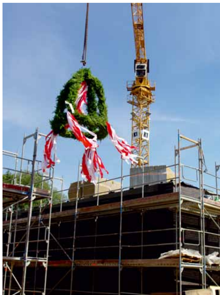
The ribbons of the topping wreath waving in the air over the new CFEL building.
