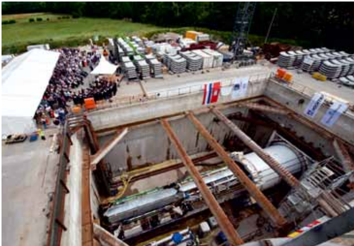
First tunnel and borer christening ceremony on the European XFEL construction site Schenefeld on 30 June 2010. In the foreground the tunnel boring machine in its start shaft. (Photo: European XFEL)
