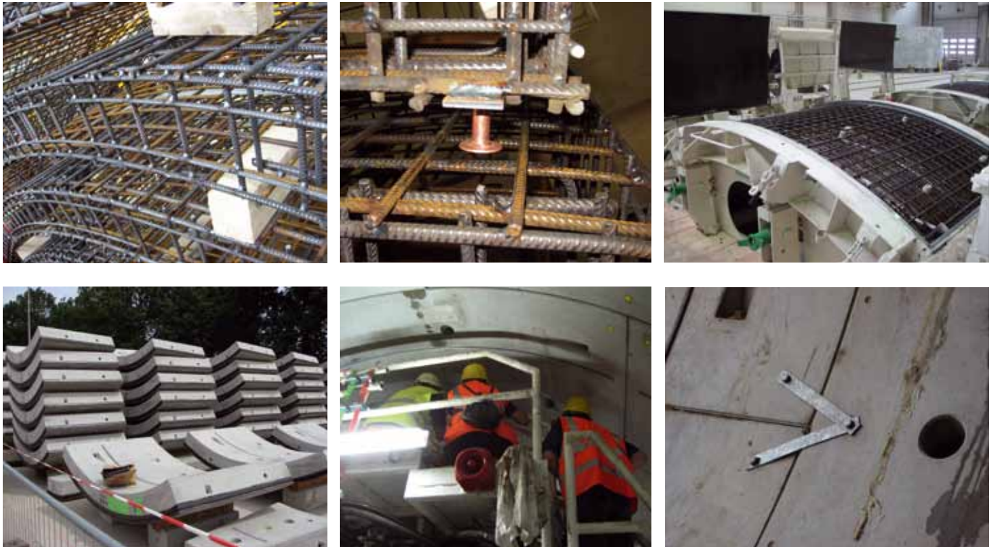
Figure 2 Inclusion of the tunnel steel in the European XFEL facility ground: 1 Steel cages – 2 Ground connector – 3 Tubbing mould – 4 Produced tubbings – 5 Tubbings in place (with yellow grounding points) – 6 Connected tubbings
