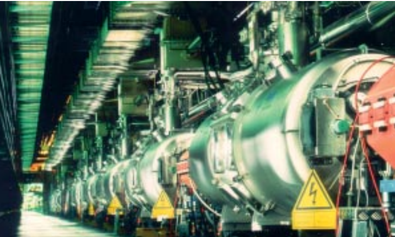
In the HERA tunnel: the superconducting resonators of the electron ring.
