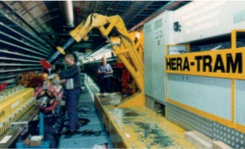
With the help of the "HERA tram," the new magnets, which weigh several tons, are transported and set up in the tunnel.
