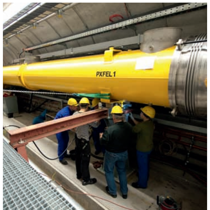
● Each accelerator module contains eight superconducting cavities cooled to minus 271 degrees Celsius.
