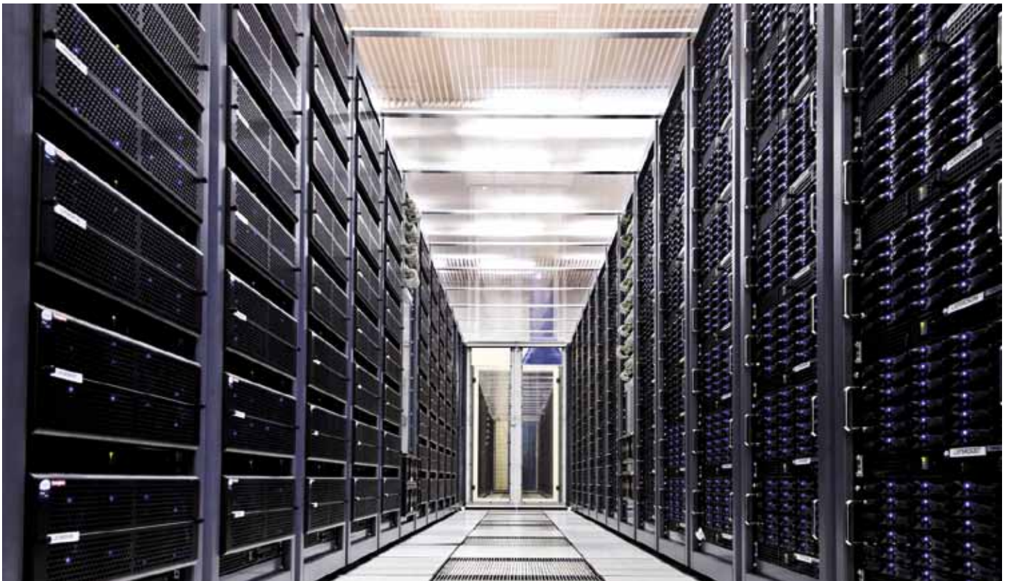
● The CERN computer centre in March 2008
