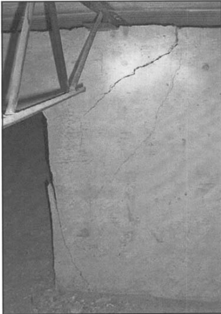
CRUMBLING FOUNDATION Chinle Boarding School, Arizona
