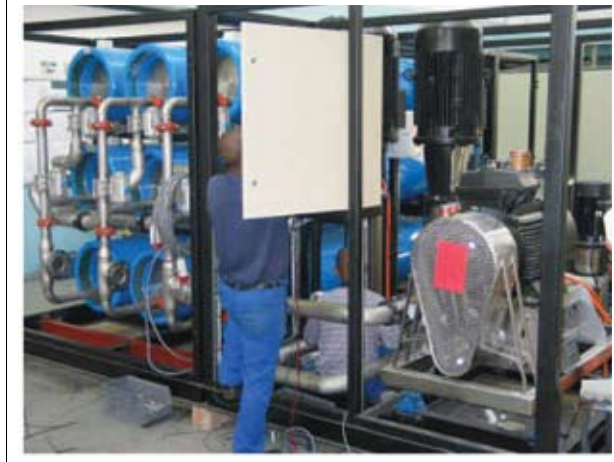
FIGURE 6 A 1 000 m 3 /day RO assembly (courtesy Graham Tek PTY)
