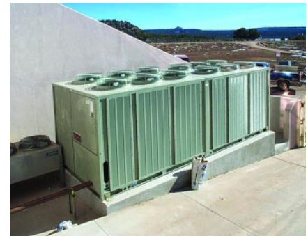
Updated heating and ventilation system
