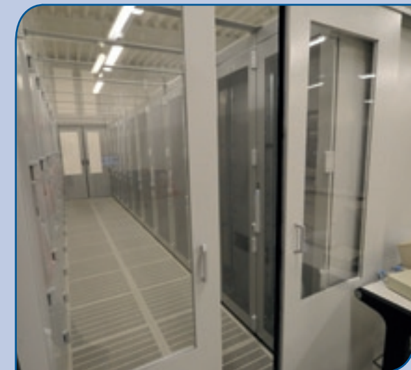
Thermal isolation of cold aisles prevents a mixture of airflows and improves efficiency of the air conditioning and cooling.
