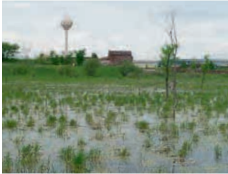
May 2001 photo of S-5 during the first season of flooding after installation of the dike and water control structure.
