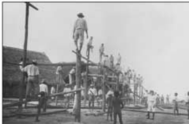
Workers erect building in Dacca, 1924. Sethi Khan, Calcutta, Benares. Photo by A. J. Hayat, Cornell.
